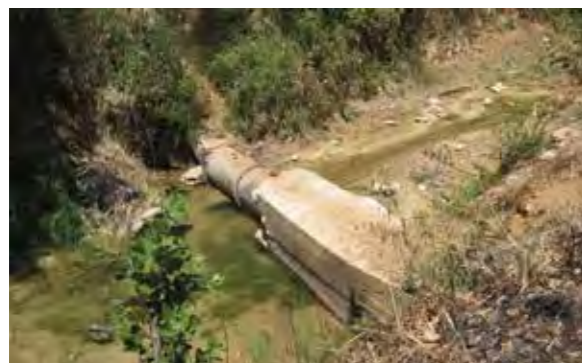
© Destroyed water duct.
